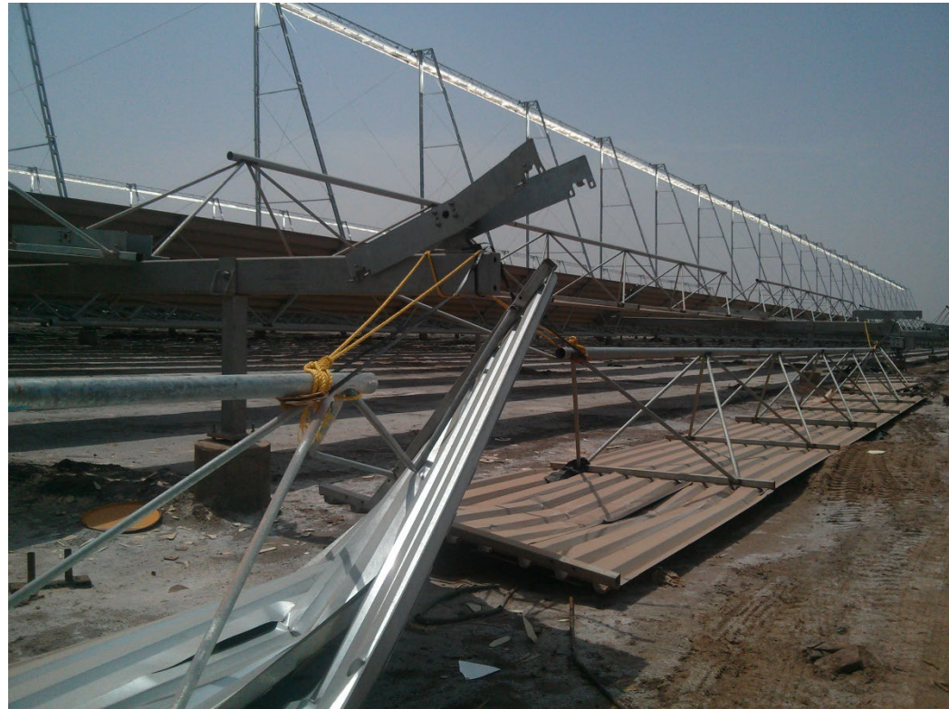
Solar Panels Destroyed by Wind
